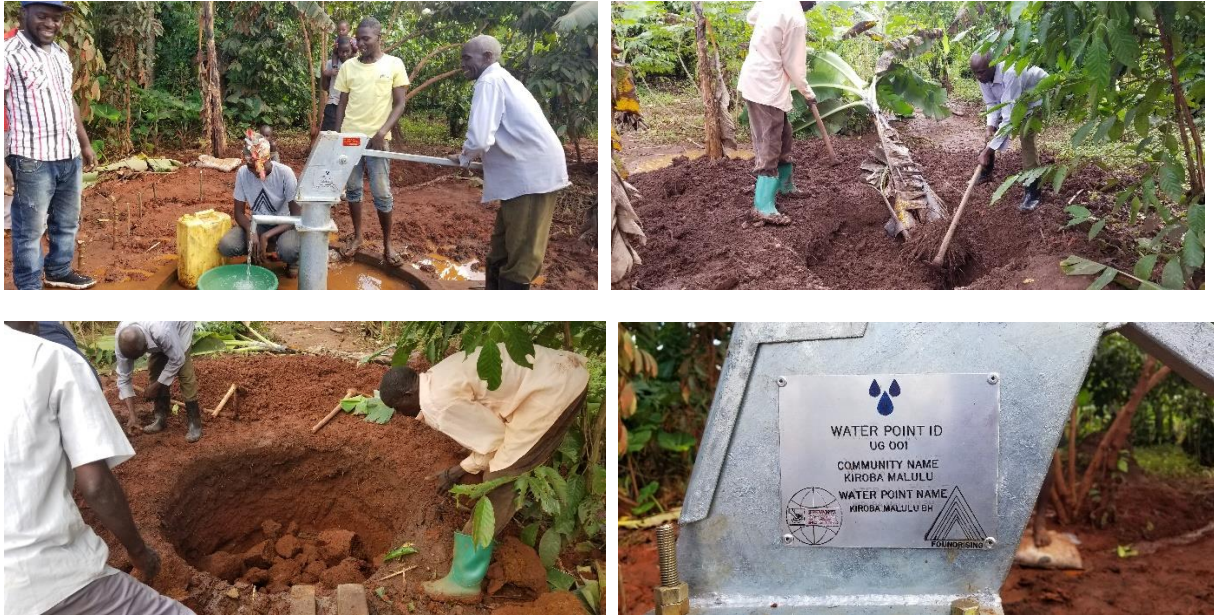
Figure 8: a community member pumping after installation and guiding the community on soak away pit
