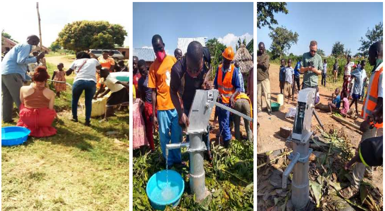
The above photos shows borehole pump testing and borehole installation in Buyende District.
