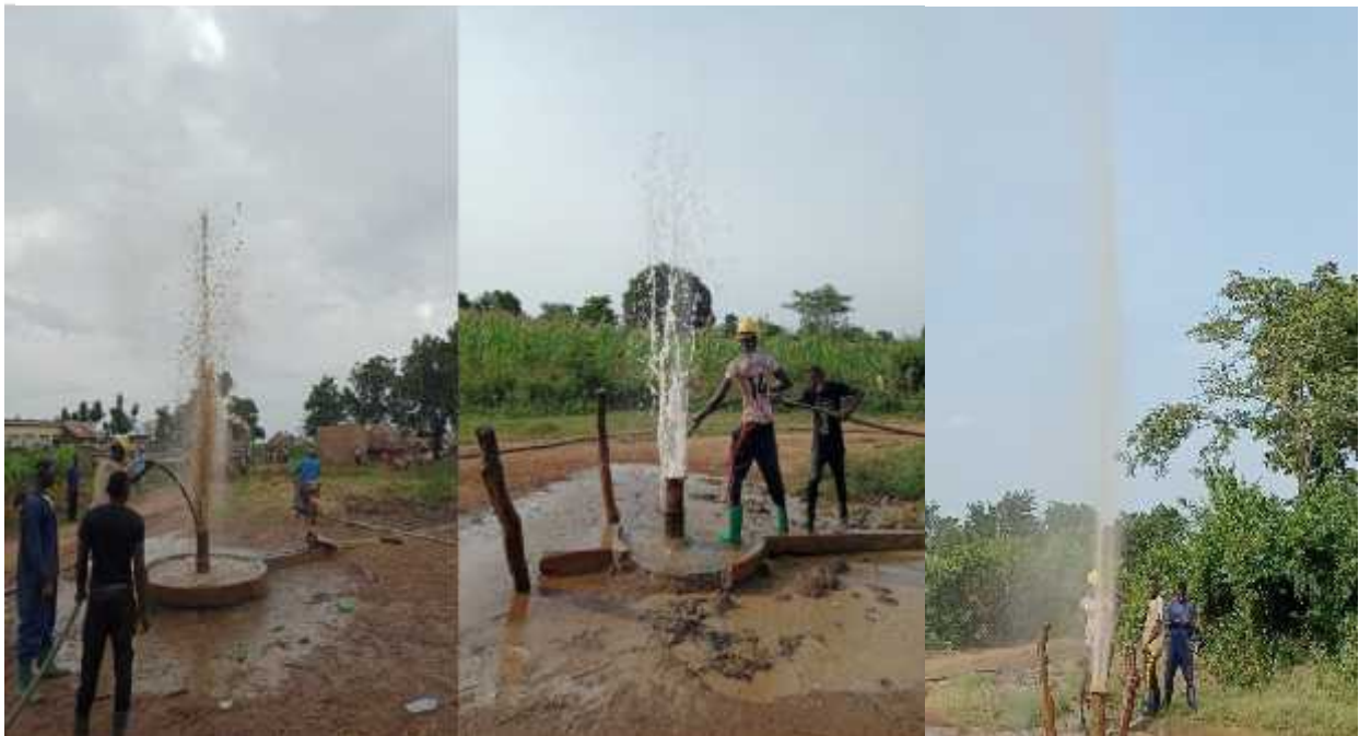
Photo showing borehole flushing in Nsonko, Kakooge and Kiribairya Villages in Buyende District
